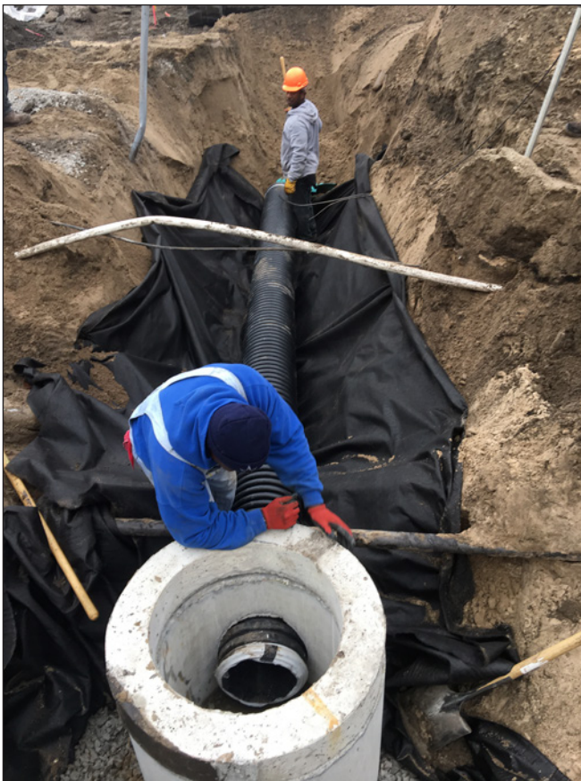
Figure 9. Photograph showing installation of perforated plastic pipe and concrete drop-down structure in the rain garden at Gary City Hall in Gary, Indiana. Photograph by David C. Lampe, U.S. Geological Survey.
