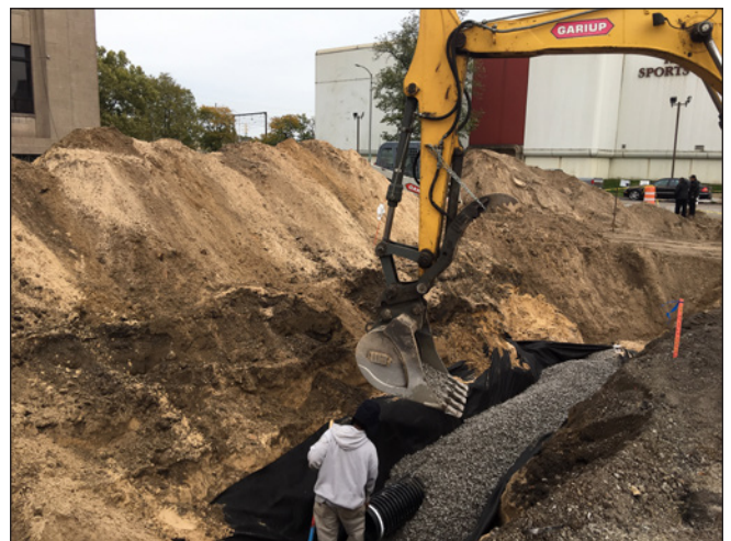
Figure 10. Photograph showing installation of gravel and root barrier around the perforated plastic pipe in the rain garden at Gary City Hall in Gary, Indiana. Photograph by David C. Lampe, U.S. Geological Survey.
