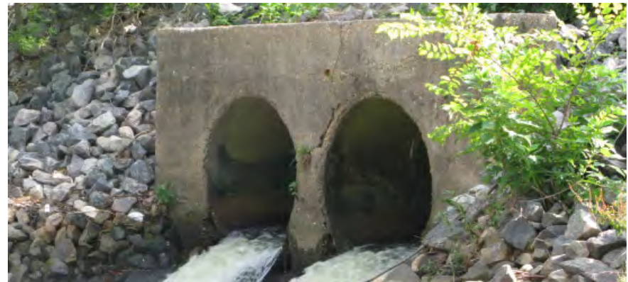
Combined Sewer Outfall (City of Richmond, Virginia)
